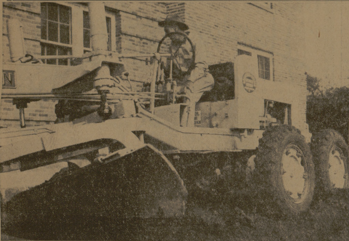
SIXTEEN TONS —Workers have been busy the past few days pushing dirt from the lawn in front of Bizzell Hall. New dirt will be added to the area and grass will be planted as another step in the overall campus beautification program. Work should be completed by the end of the week.
