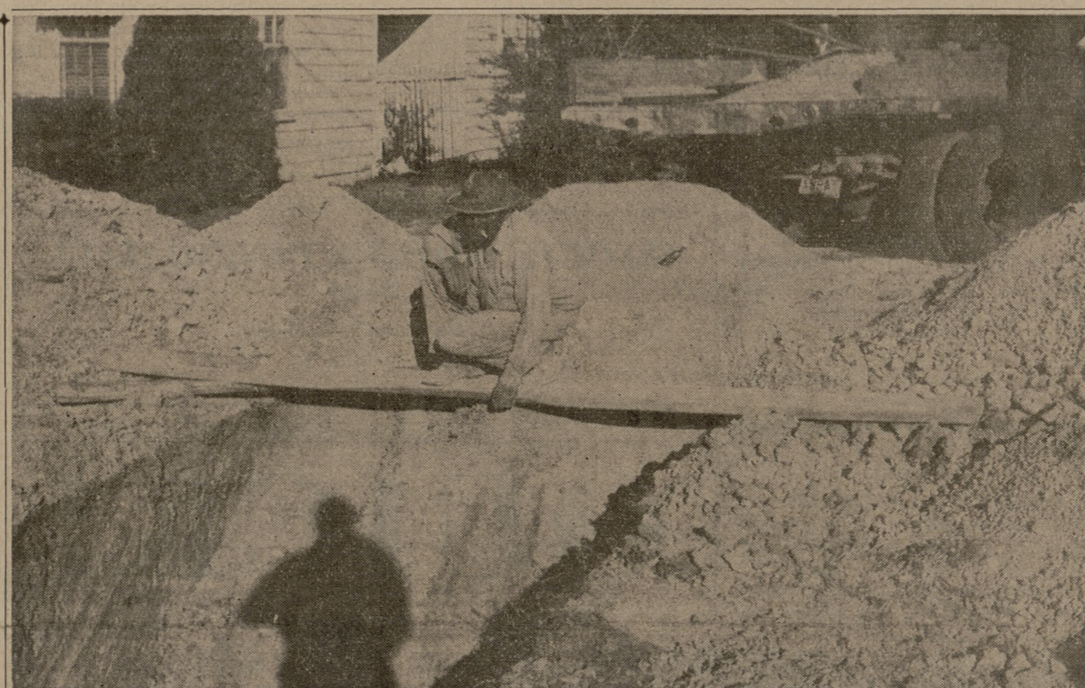
PIPELINE—The new College Station sewer line has crossed the city limits and is expected to be completed in about 150 more days. The complete system will include 80,000 feet of pipe ranging in size from six to fifteen inches. The Texala Construction Co. of Houston is doing the work.
