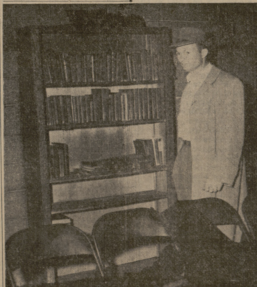
FIRE DAMAGE —The Rev. Clarence Ketch, pastor of the A&M Christian church, surveys damage done to the church building by the fire early Monday morning. Some of the damaged books in the book case may be saved. The trash on the chairs in the foreground fell from the roof.
