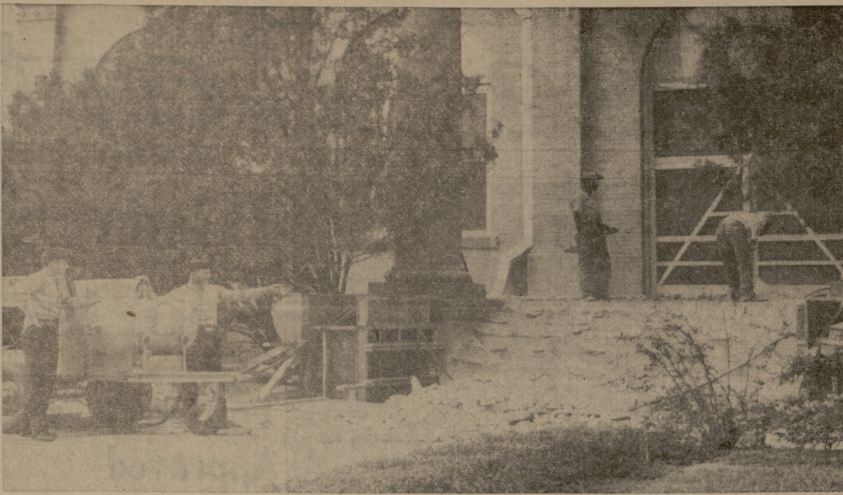
NO MORE FALLS —Tom Goldstone, left and Fred Pool watch workmen tear down the front steps of Sbisa dining hall. The steps were too steep, causing cadets to fall as they were marching up them, according to J. G. Peniston, dining hall director. He said the new steps would not be as steep. The work is a part of the renovation of the building.
