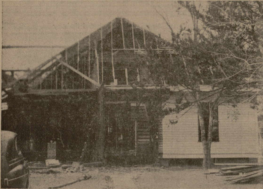
THE COLONEL'S MOVED —Workmen are dismantling this house, formerly the home of Col. Joe E. Davis, commandant, to move it elsewhere on the campus. This house is one of four along the street that are to be moved this year. Plans are not definite as to what will be built in the space occupied by the houses.
