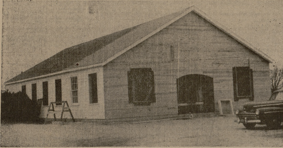
UNDER CONSTRUCTION—M. M. Cook and R. E. Logan, deacons of the College Heights Assembly of God, are doing the remodeling carpenter work on the church, above. The building is expected to be completed around Jan. 15. Jimmy Boswell, senior architect major and a member of the church, drew up the plans for the construction.
