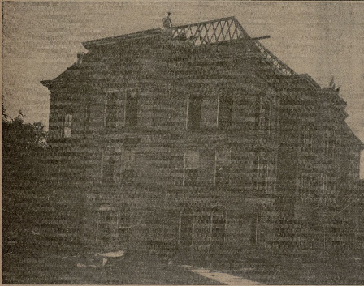
GOING, GOING—Ross hall, long-standing home of A&M's bats, bulls, and students, is being demolished. Wrecking crews start on the roof.
