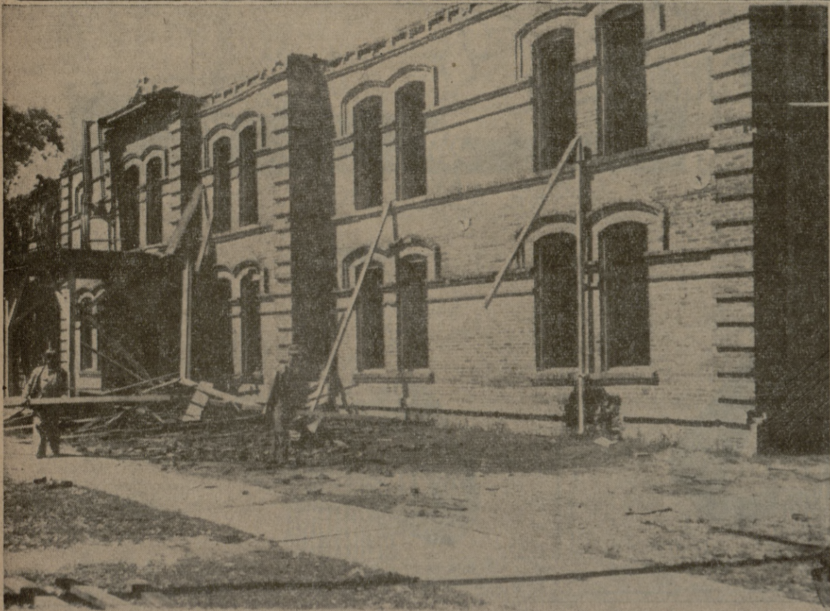
GOING DOWN—A familiar sight for the past 67 years on the A&M campus is now being torn down. The building was built as a result of poor management in the mess hall.
