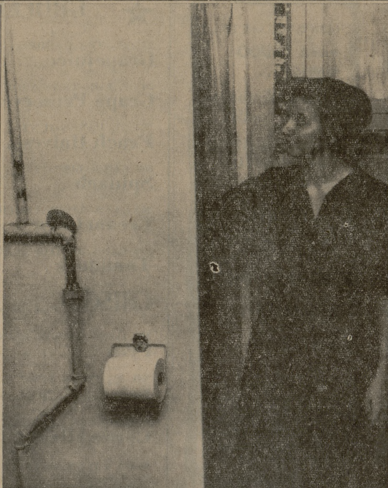
LOOKS GOOD—Mrs. Mary Norris inspects the new showers now being installed in the College View apartments. The new showers are part of a $140,000 improvement program for the apartments.
