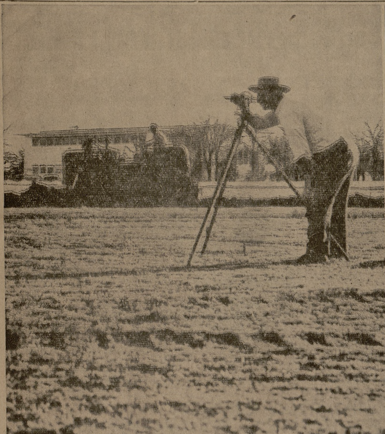
CITY'S NEW SCHOOL —Work started yesterday on the new school building for A&M Consolidated high school. C. L. Andrews of Andrews-Parker Inc., general contractor, surveys the location while a bulldozer begins leveling. The Consolidated gymnasium is in the background.
