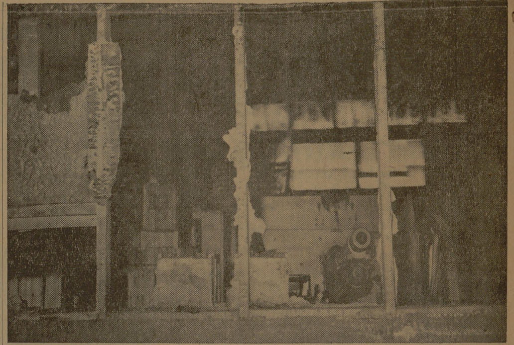
A photographer got this close up view of damage done to the military property custodian's office building and warehouse by a fire Friday night which completely gutted the tin frame structure. Rifles, artillery pieces and other equipment were saved, although records of the custodian were either completely or partially damaged.
