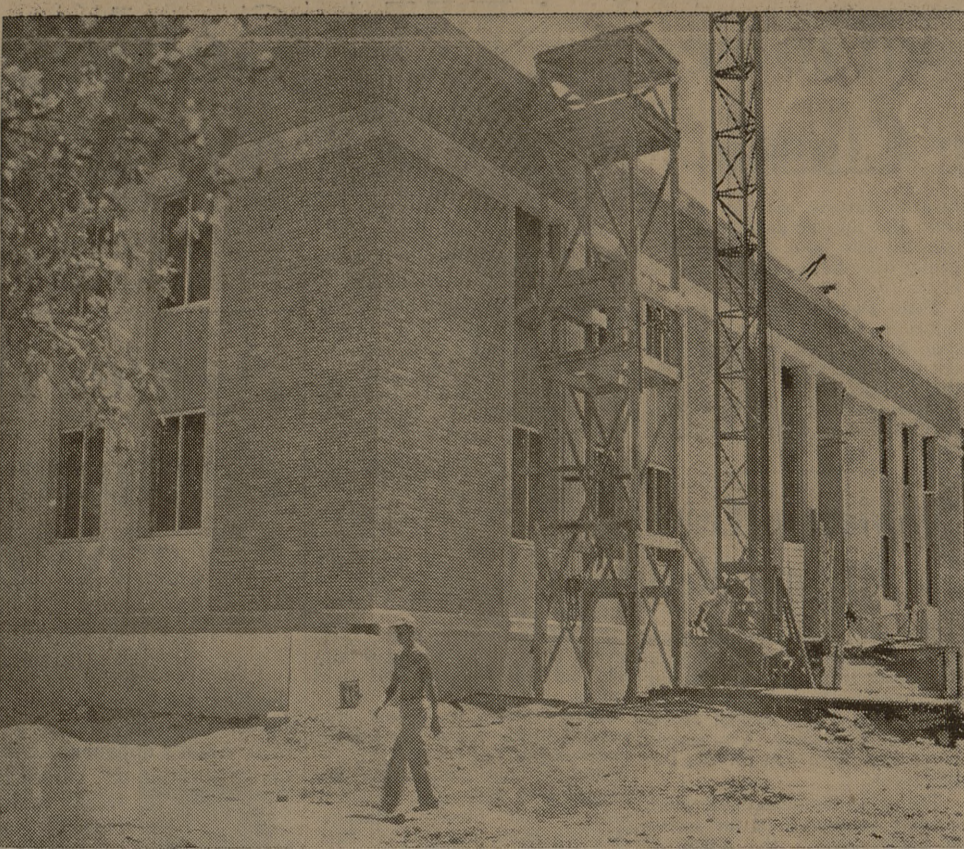
The new college Administration Building gets finishing touches on the outside as workmen hurry to complete the interior by late October or early November. Offices of the deans and president, as well as the Fiscal and Registrar's Offices will occupy the new structure. A recent bricklayer's strike has held up masonry work for over two weeks, however the men returned to their jobs Monday.
