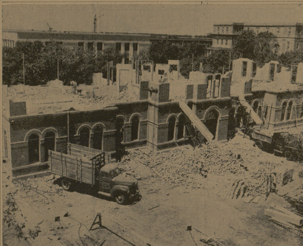
As the new building to house college administrative offices rises in the background, old Foster Hall is gradually becoming leveled as workmen complete destruction of the second floor of the
