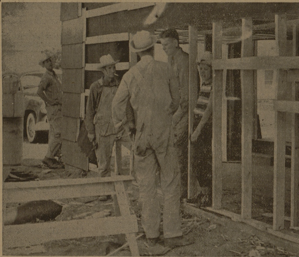
Workmen immediately began to repair the home of Major T. F. Peters which was damaged yesterday morning after a Bryan Police Department patrol car tore into the structure. The Major's automobile is seen in the far left of the picture. Estimated damage to the car and house was around $500. Workmen are employed by Smith-Hawk Company.
