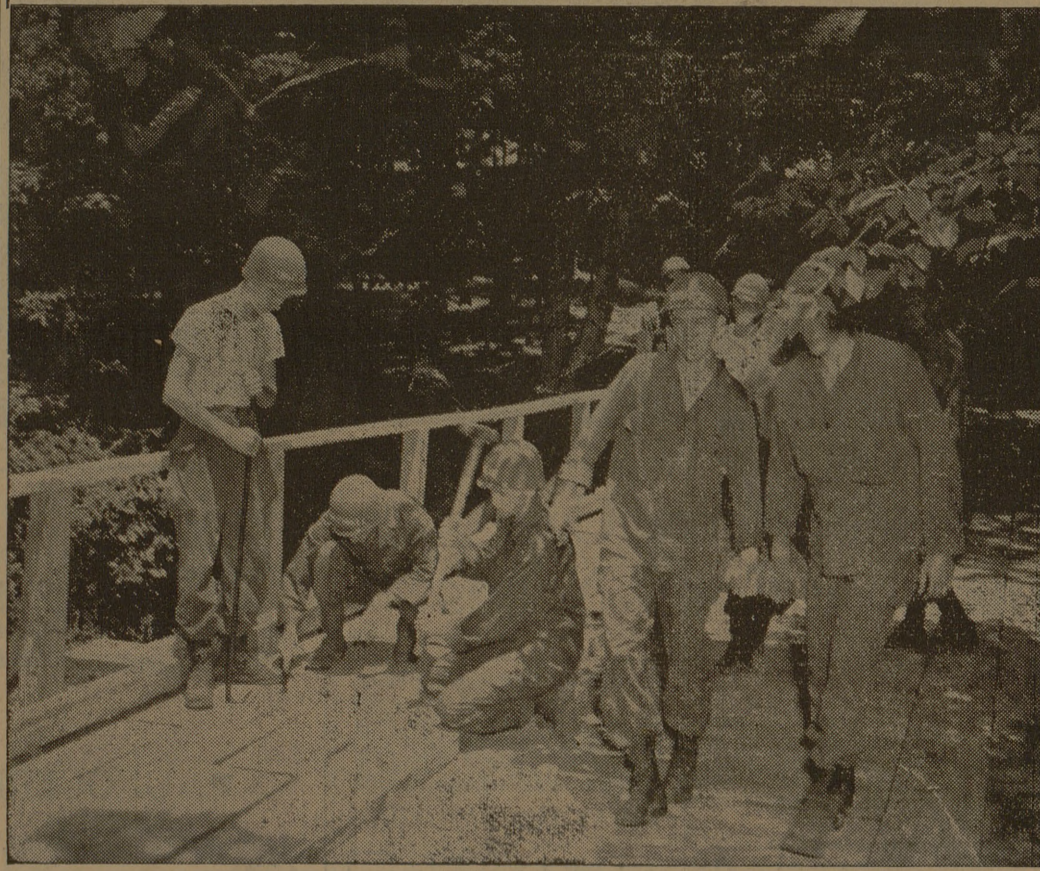
Cadets Hershel G. Truelove, Blue Ridge; James E. Hulse, Houston; and James O. Atwell, Jr., Paris; are shown nailing flooring of a temporary military bridge at the Corps of Engineer's ROTC
