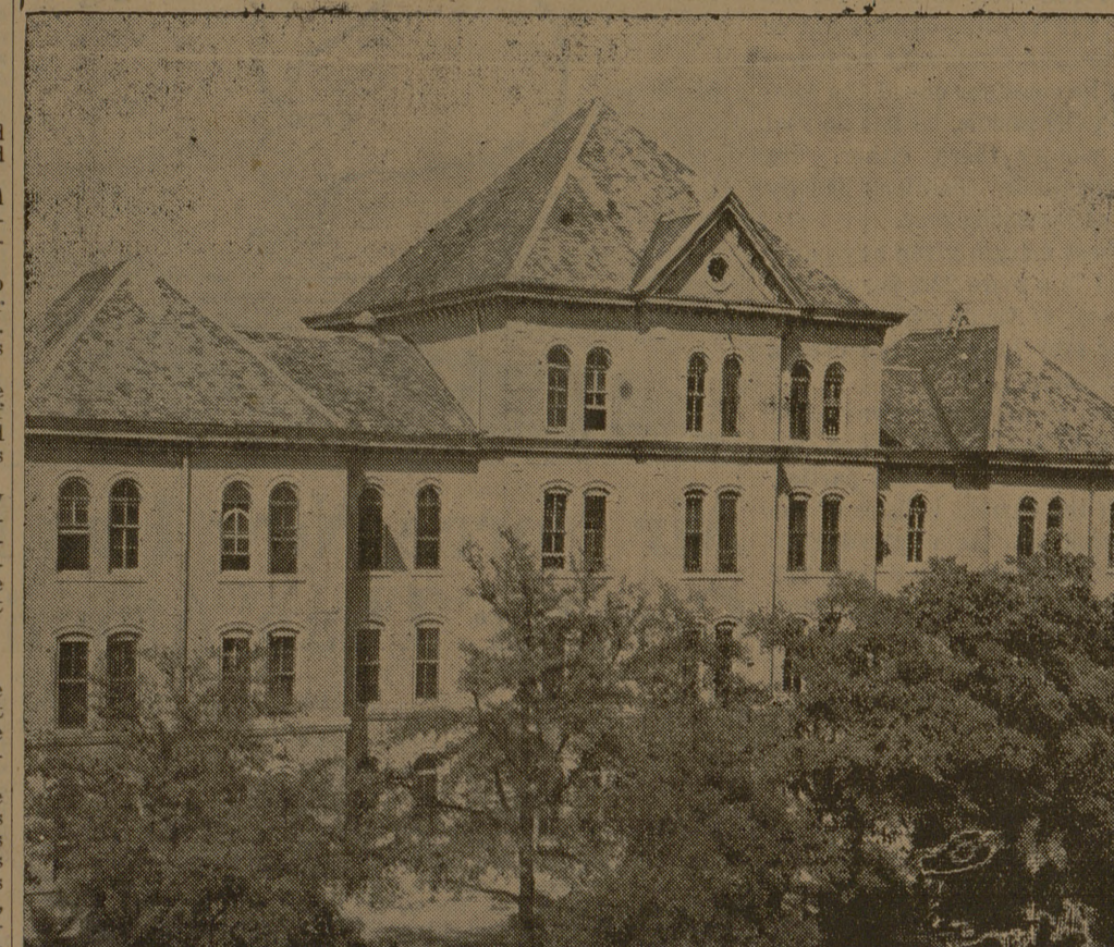
Pigeons and other creatures occupying old Foster Hall were searching for a new home this week as workmen began tearing down the 52-year-old building. Constructed in 1899, Foster was originally used as a dormitory, and after age set in, was converted into storage space.
