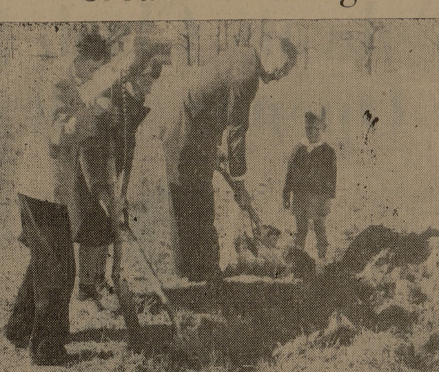
The Rev. Norman Anderson, pastor of the A&M Presbyterian Church, breaks ground for the new Sunday School Building. The official ceremony was held Sunday.
