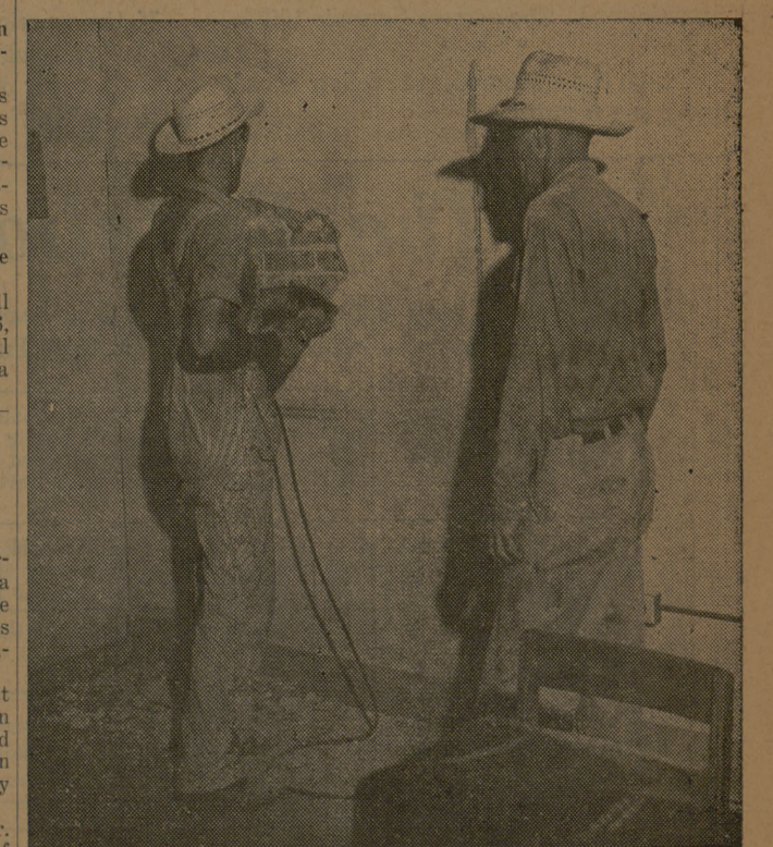
Keeping the college's physical plant in top-notch condition is quite a job, and these are some of the men who do it. Drilling through a wall in the Student Apartments offices in Goodwin Hall, this crew has joined the offices with a new door. All over the campus this summer, B&CU men are making minor and major repairs and changes in anticipation of a crowded campus this fall.
