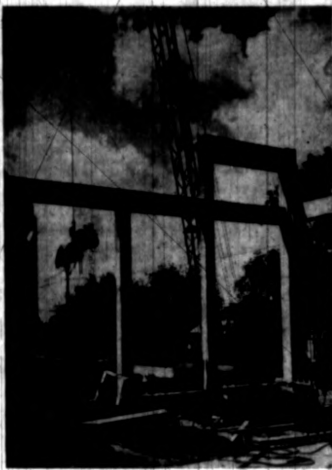
College Station's new A&M Methodist Church building now shows only a skeleton framework, but it won't be long before another beautiful church decorates the North Gate area. A worker gets a free ride from the crane operator, as they prepare to place more of the structural steel atop the building.
