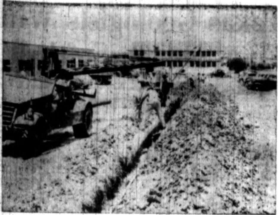
"The pipes go down" as work on the water main to the Feeder Breeder Station west of the college's new wells continues. At present, pipes are being laid through the North Gate Area to the reservoirs already constructed.
