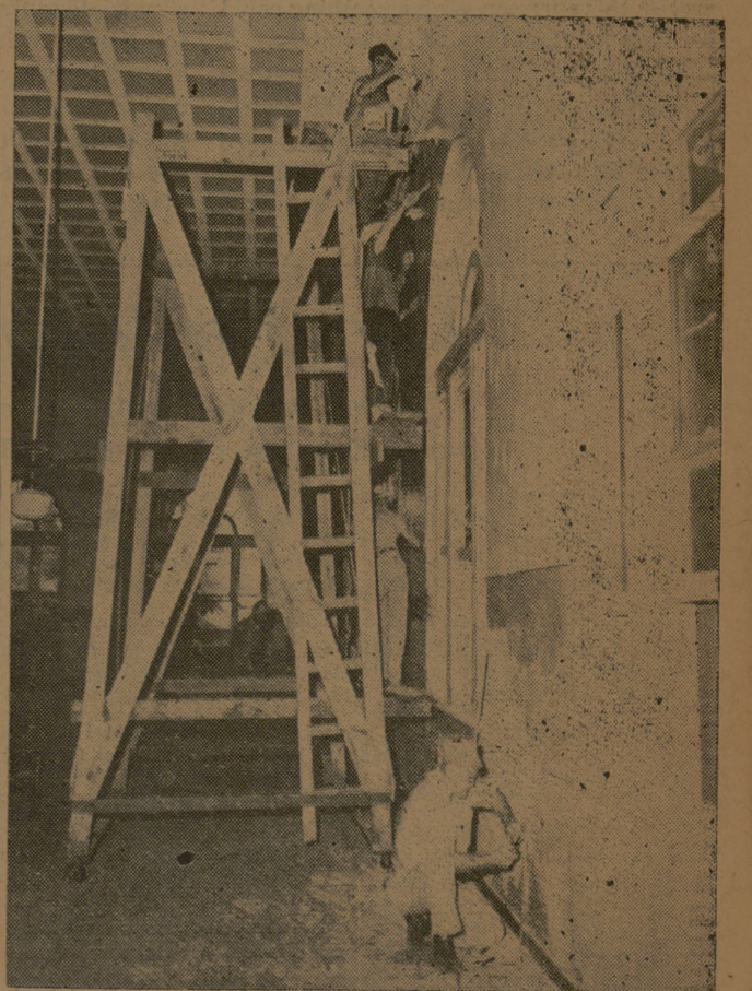
The main dining room of Sbis Hall is getting a face lifting. Workers are replastering and painting the walls. The dance floor is being sanded and refinished.
