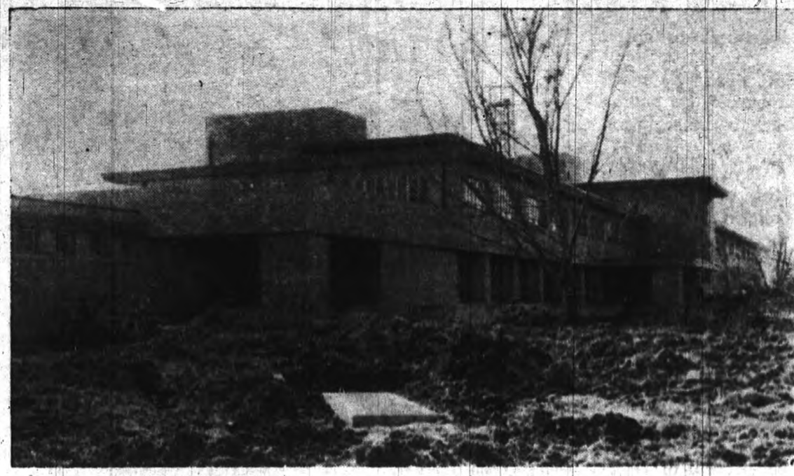
Progress on the Student Memorial Center is rapid, as shown above. The structure is due to be completed Sept. 1. It is part of the $6,293,000 construction program now underway here.
