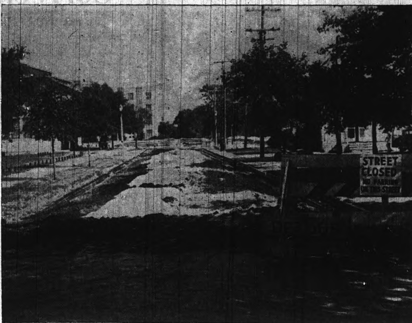
Street repairs begin on the campus. The corps area streets are the first to be improved in a program scheduled for completion by the opening of the Fall term.
