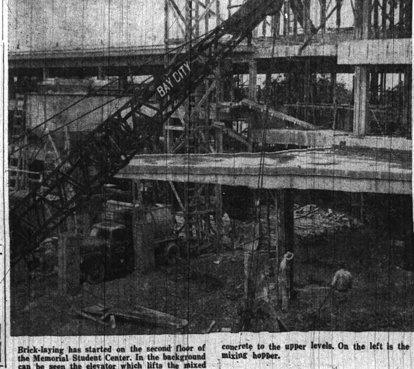
Brick-laying has started on the second floor of the Memorial Student Center. In the background concrete to the upper levels. On the left is the mixer hopper.
