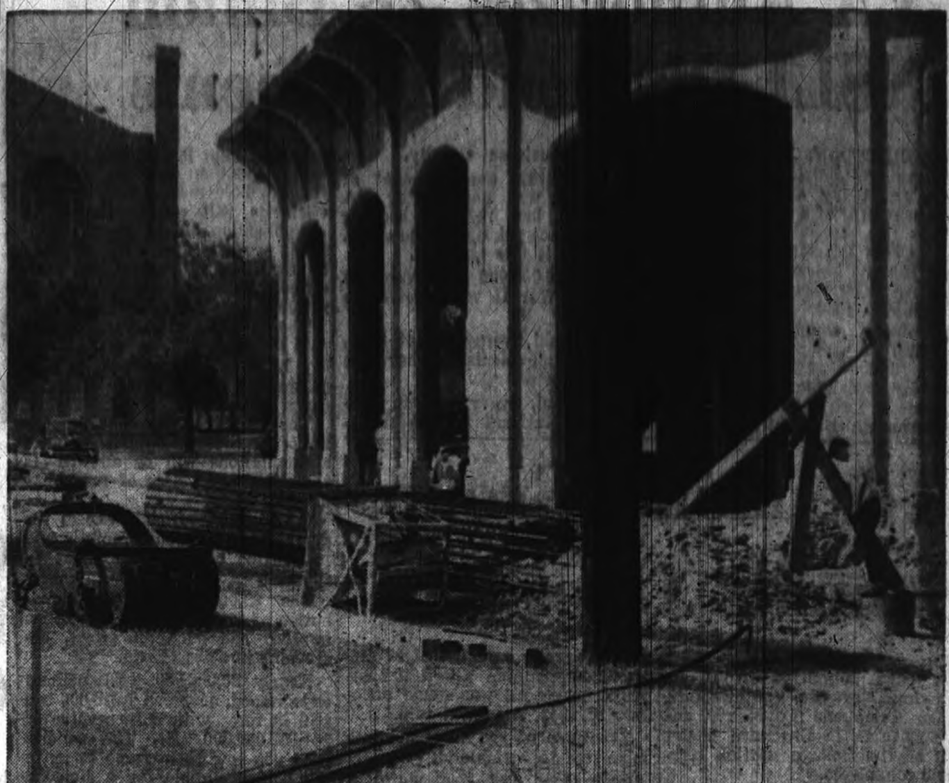
One of the student workers on the Kyle Field lighting project bails out the recently excavated hole for the West, fifty yard pole. The workmen struck water at around twenty feet and had a budding water well on their hands during the heavier rains.
