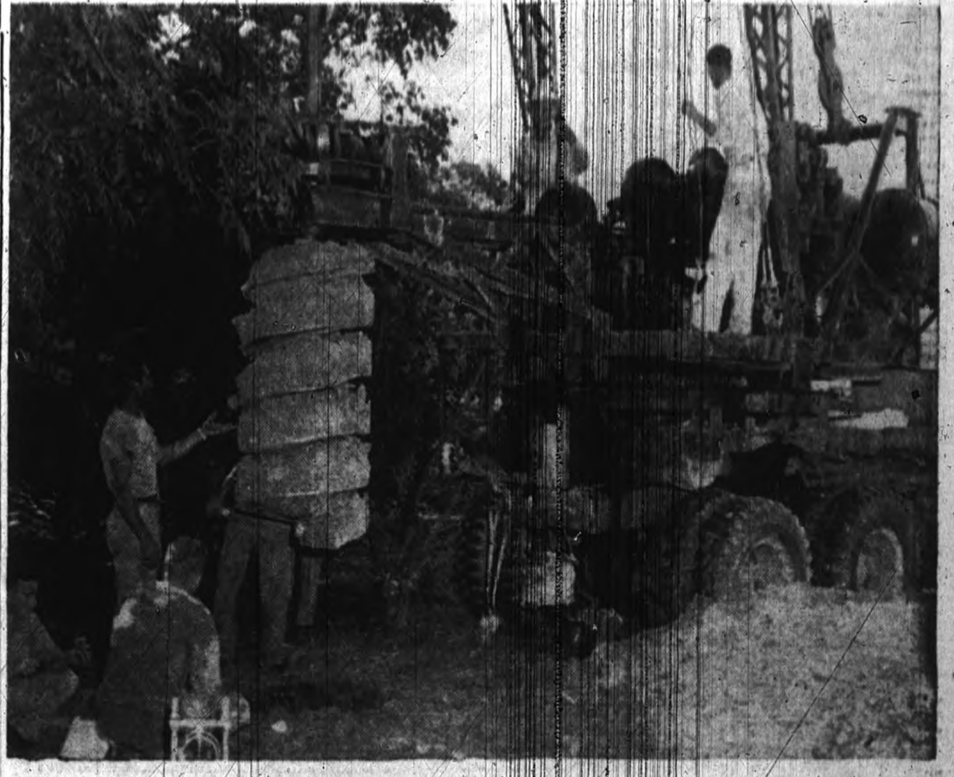
A big borer from the Watson Foundation Company of Dallas digs in behind the Science Hall as pros and students of the CE department look on with respect and admiration. In the College Station heat, they decided, the machine beats pipe and shovels by several miles, leagues and yards.
