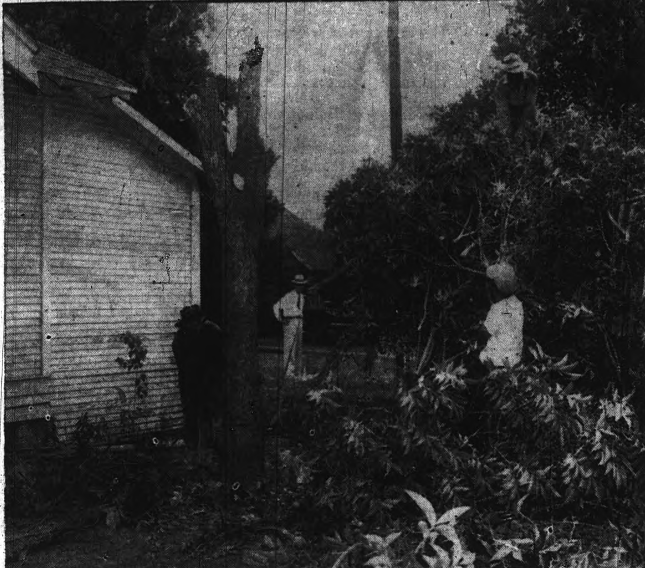
HENRY HATCHET "turns up the first shovel of dirt" for the MEMORIAL STUDENT CENTER with the aid of an axe. Though the occupants of the houses have moved out, clearing of the trees is the first tangible move in the construction program. SIPPLE YBERRA reaches the limbs up to WALTER BANK on the truck. The house will be moved to the site of the First Christian Church at the South Gate. JESS CONLEE, contractor, is doing the moving. B. D. MARBURGER, manager of utilities, is looking on.
