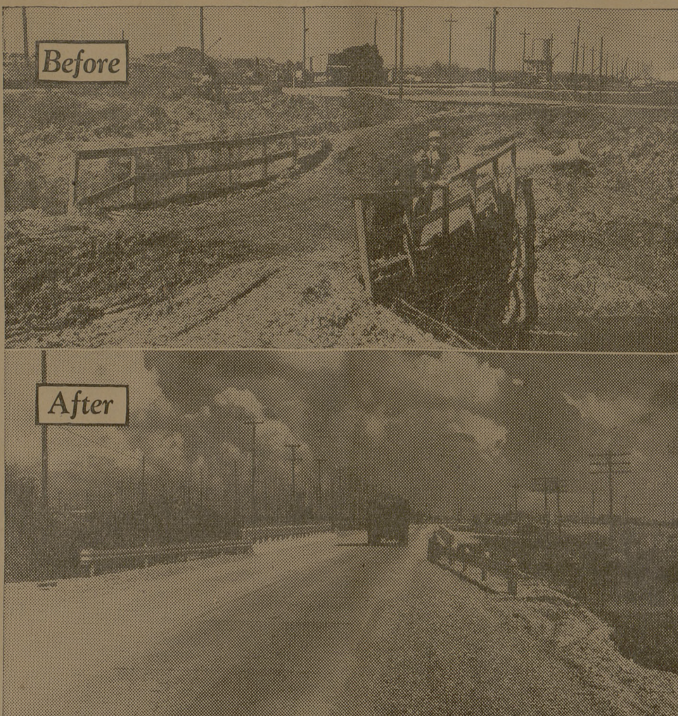
These pictures, taken from the identical spot six months apart, illustrate graphically how WPA workers transformed a muddy and virtually impassable access road to Camp Wallace, Galveston County, into a high speed and durable concrete highway. In Texas WPA has built and improved 1,423 miles of roads classified by the War Department as of strategic military importance.
