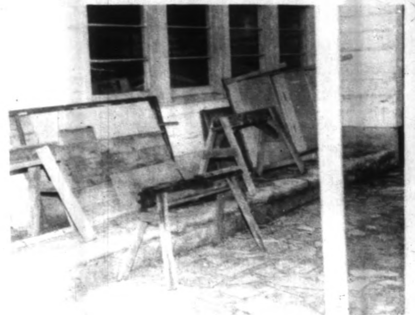
This is a view of one of the older six classroom buildings now being used for storage and maintenance work. The present Bond issue proposes to demolish the building; I say it can be restored and used, but the maintenance personnel certainly need a more adequate place for storage and working.
