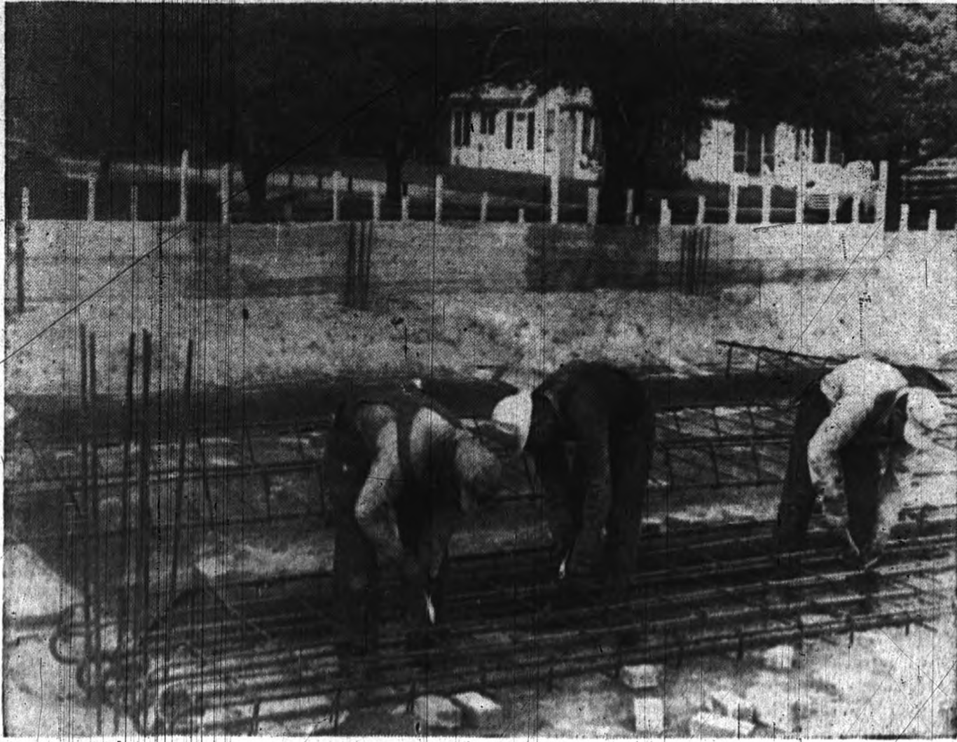
Workmen wire up the steel reinforcement forms for the supporting columns of the new Student Union bowling alleys. The pin boys' pits will be located against the wooden forms in the back-ground.
